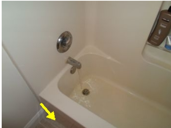
Caulking needed at tub where it meets the floor.
