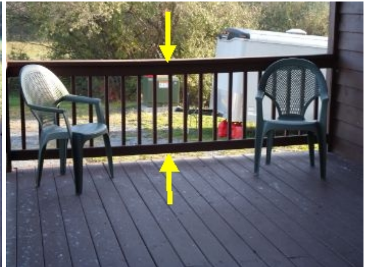
Balusters spaced too far apart.
