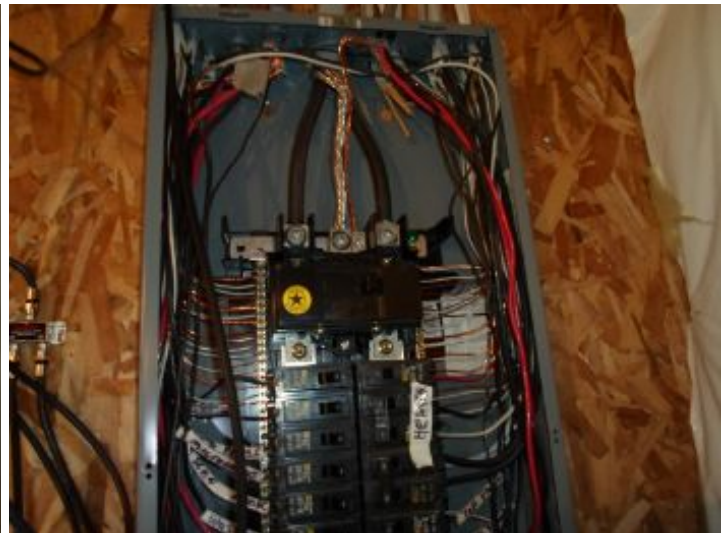
The wiring within the panel appeared satisfactory and functional, at time of inspection.
