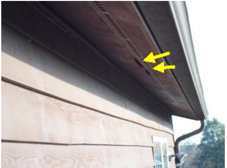
Warping soffits is allowing bees and insects to penetrate into the house.
