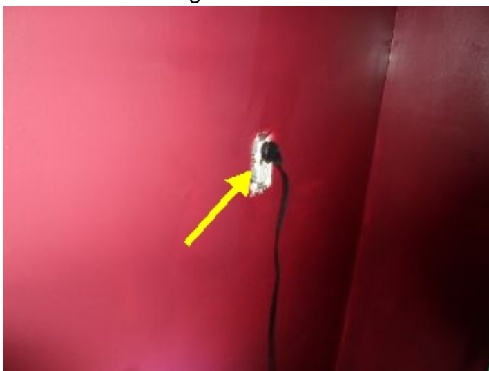
Missing plug cover needs to be fixed.
