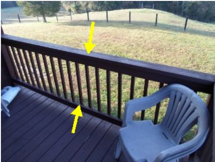
Balusters spaced too far apart.
