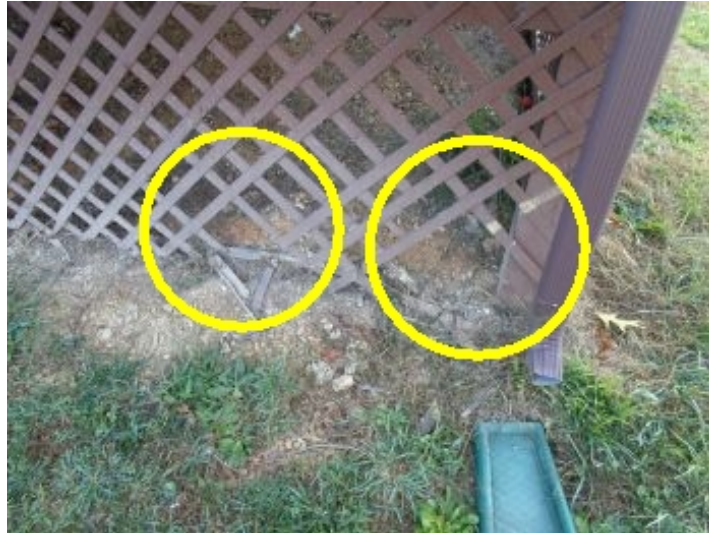
Lattice is broken in some areas.
