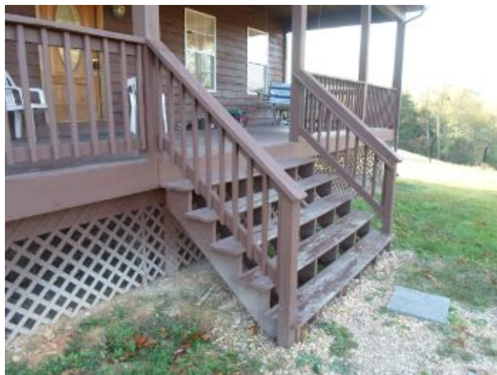
Appeared functional, at time of inspection.
