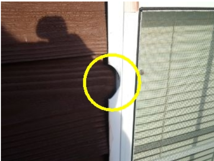
window trim is damaged
