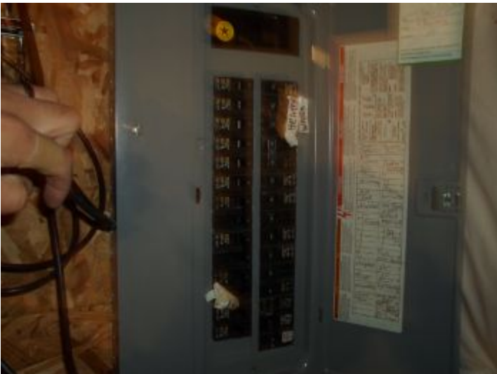
The wiring within the panel appeared satisfactory and functional, at time of inspection.
