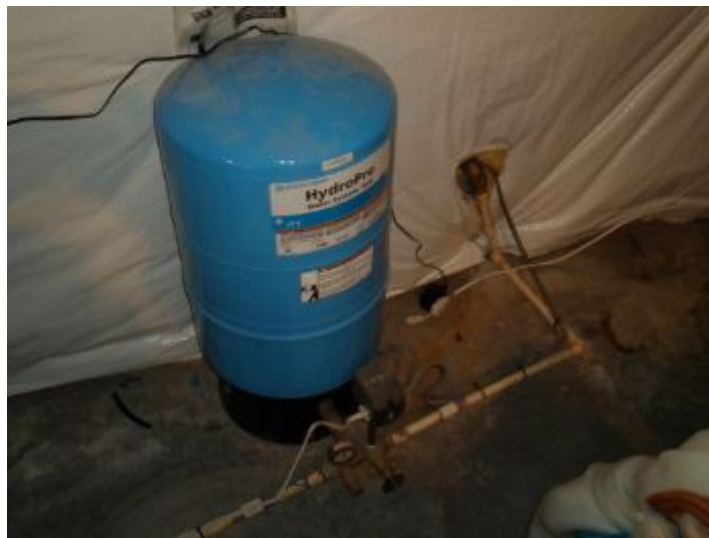
Appeared functional at time of inspection.
