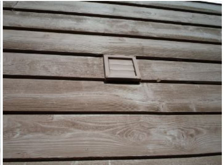
Appeared functional at time of inspection
