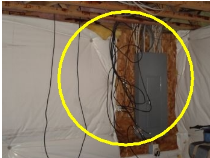
Loose cable/phone wires. Have reviewed.
