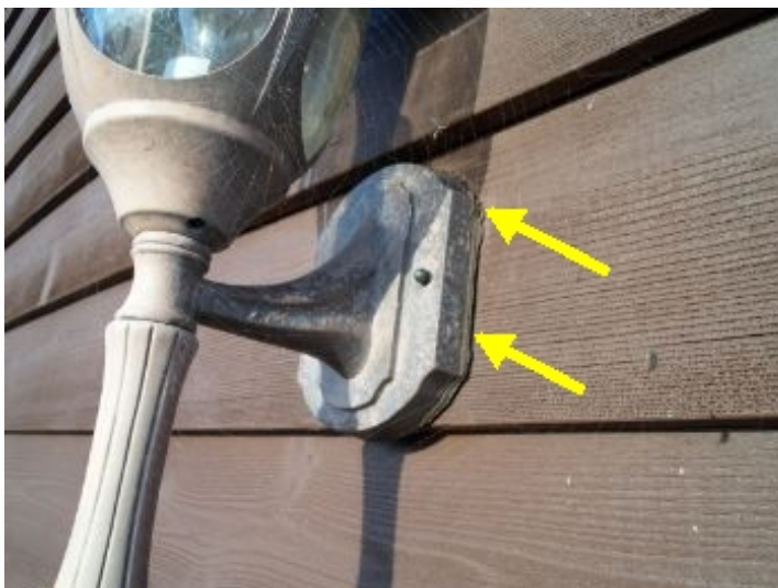
Exterior light fixtures are loose.
