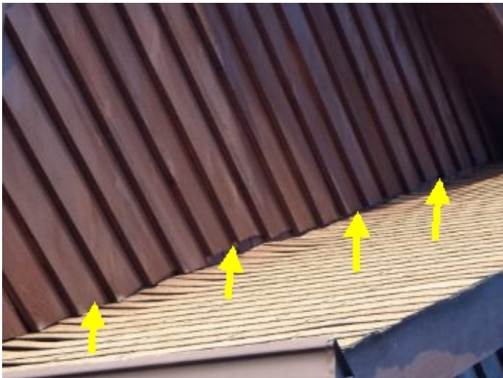
Uneven gaps going up the roof line.
