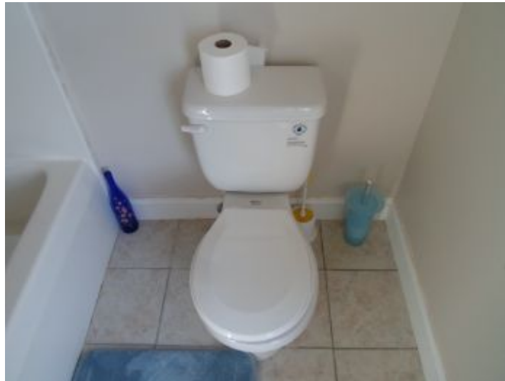
Operated when tested. Appeared functional, at time of inspection.
