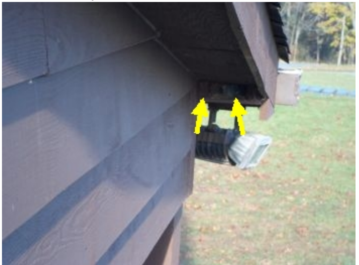
Warping soffits is allowing bees and insects to penetrate into the house.
