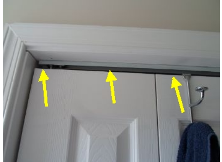
Doors damaged/missing and not installed correctly
