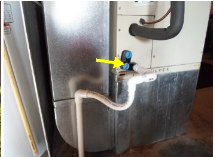
Secondary overflow isn't plumbed and doesn't have an over flow cut off switch.
