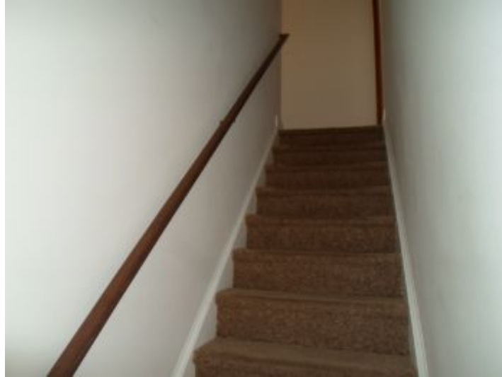
Appeared functional, at time of inspection.
