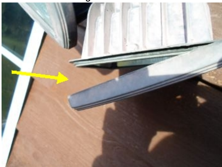
Exterior light fixtures are loose.
