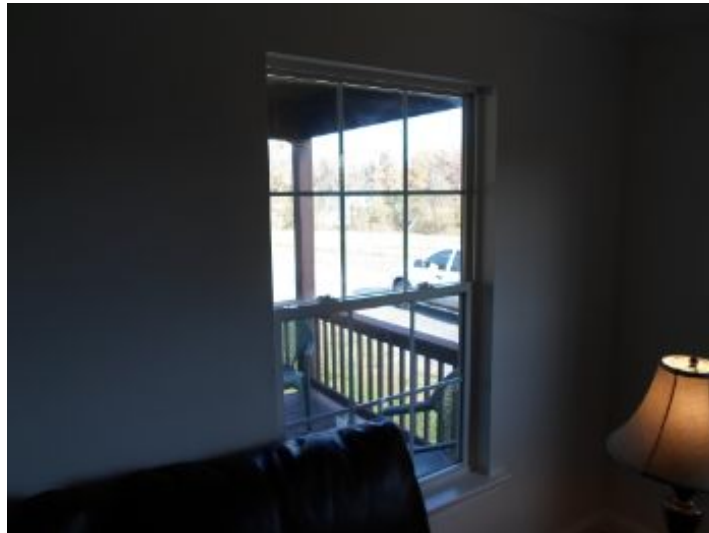
Some windows do not operate as designed.
