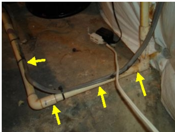
Service pipe from well is unsupported and if stepped on would break off.
