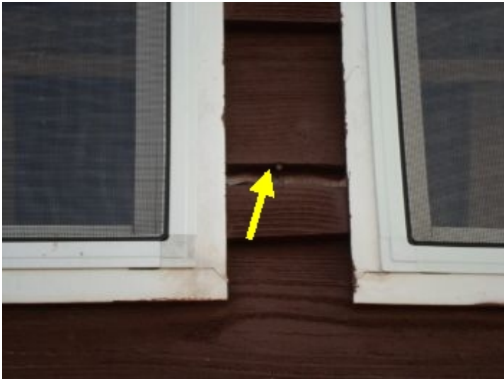
deteriorated materials needs to be maintained with caulk and sealer.
