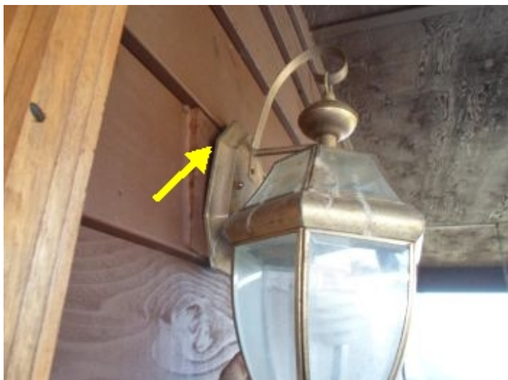
Exterior light fixtures are loose.
