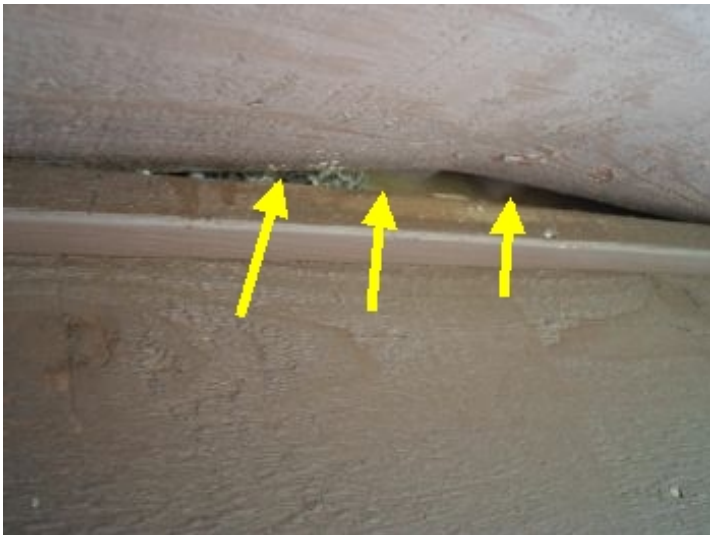
Warping soffits is allowing bees and insects to penetrate into the house.
