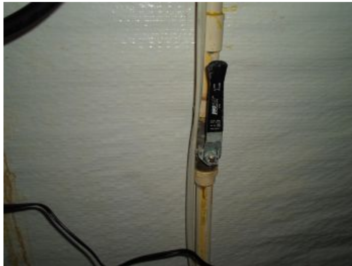
Appeared functional at time of inspection.
