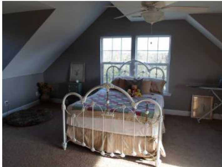
Some paint and drywall touch up needed.
