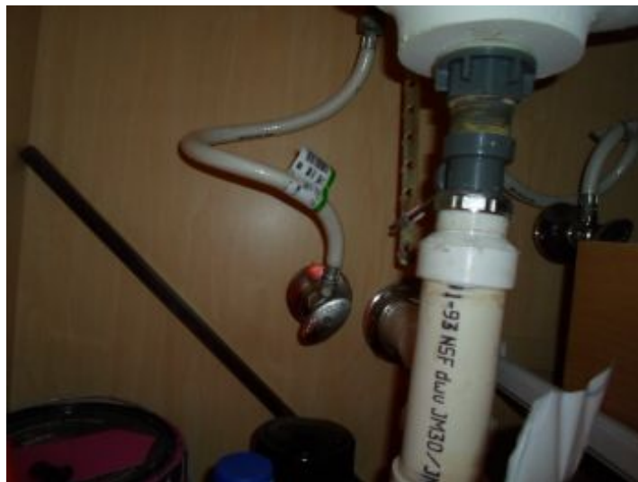
Water was run through the fixtures and drains. Functional flow was observed. Functional drainage was observed.
