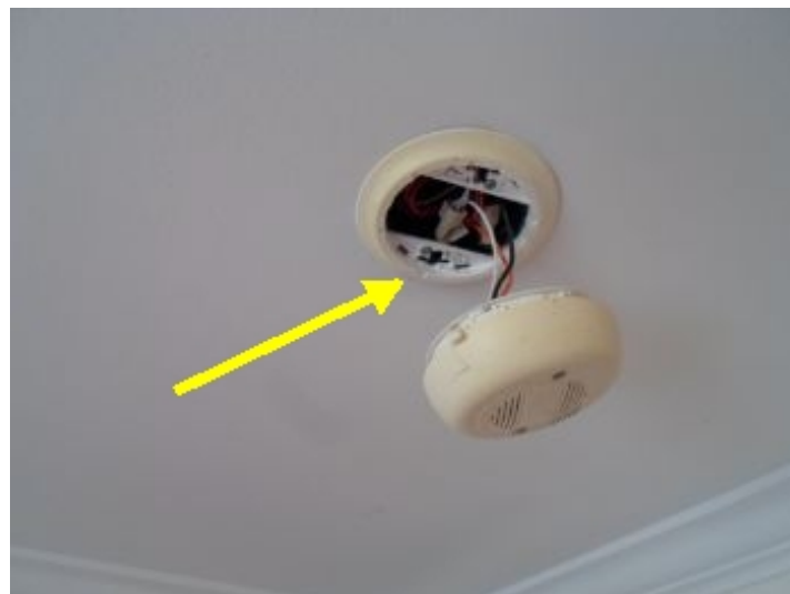
Smoke detector is loose and hanging from the wires.
