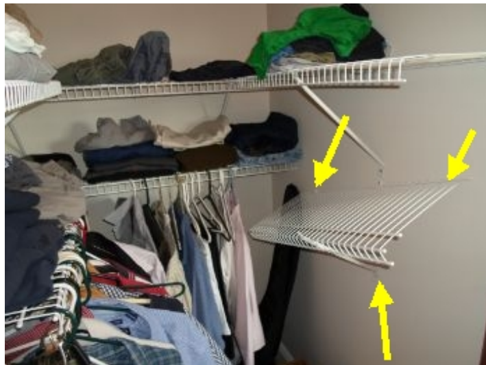
Shelves in closet damaged/missing
