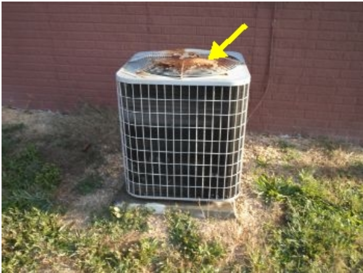
Rust/Stained at exterior condensor.
