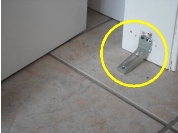
Doors damaged/missing and not installed correctly
