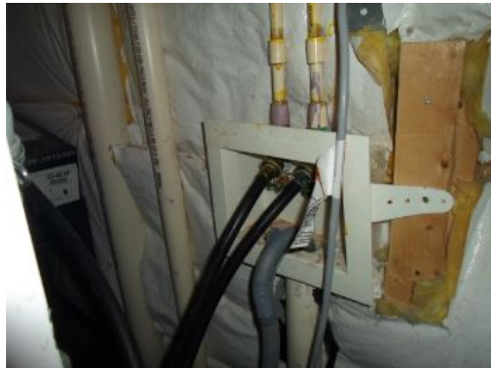
Recommend upgrading washer hoses to braided type lines.
