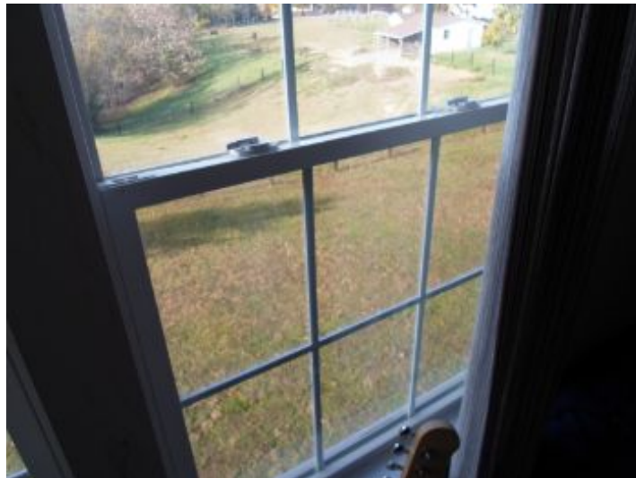
Does not operate properly
