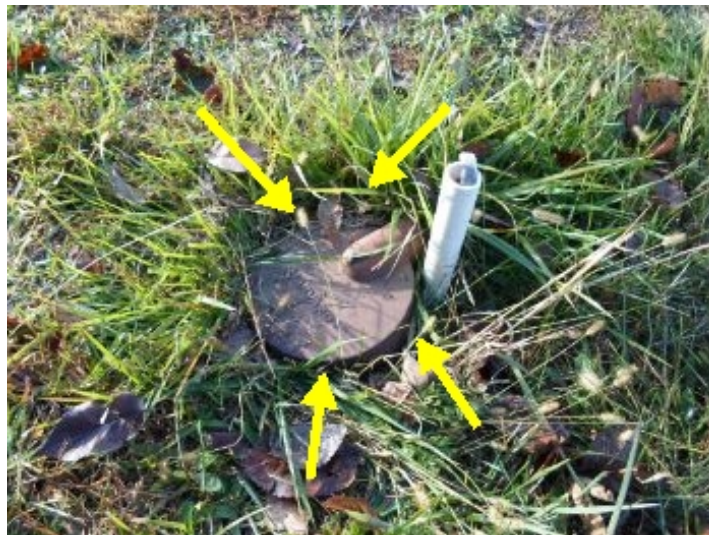
Well pump casing does not come out of the ground high enough. Rain water run off is contaminating the well water.
