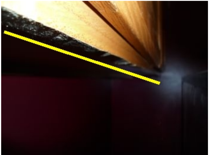
Cabinet over top of the fridge has been chopped up to make it fit.
